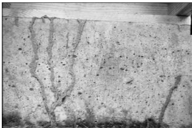
Fig. 1. Traces (mud tubes) of subterranean termite penetrated the foundation concrete slabs constructed from sand only.
